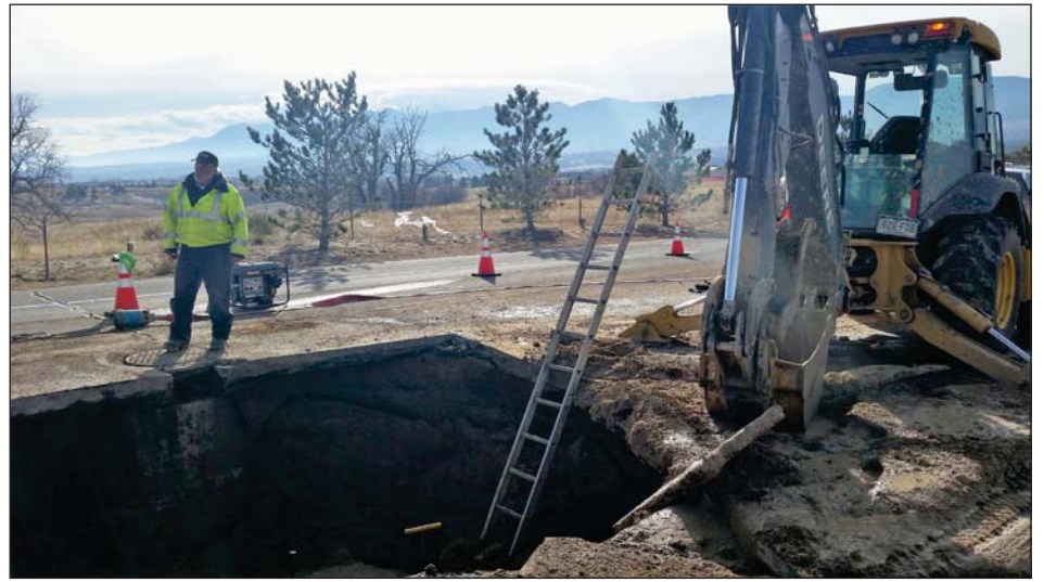
Above: On Jan. 6, the town of Monument announced that westbound Second Street between Highway 105 and Old Denver Road had been closed Jan. 4 and 5 to repair a water main leak first spotted the morning of Jan. 4. The town’s Water Department and Streets Department staff worked overnight in wind-chill as low as minus 22 degrees F to repair the leak by Thursday morning at 5 a.m. Public Works Director Tom Tharnish said the break and repair did not affect any water customers and that the excavation site would be paved when weather conditions allowed. Contact Tharnish at ttharnish@tomgov.org or call 719-481-2954 with questions. Photo courtesy of the Town of Monument.
