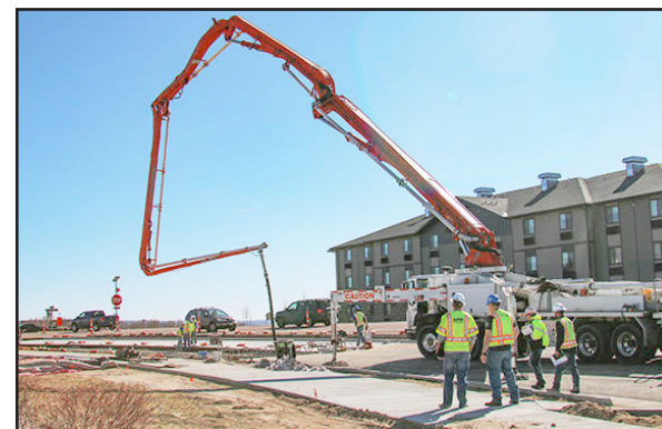
Above: A pumping truck pours concrete as work continues on the Struthers/Gleneagle intersection project Photo courtesy of Crystal Peak Design
