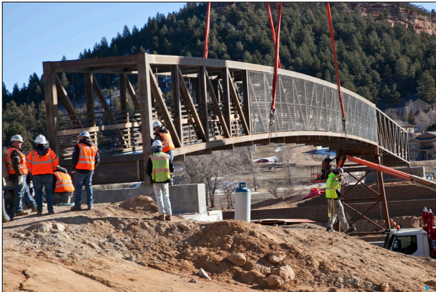
Above: On January 7, SEMA Construction Inc. installed the two sections of the bridge manufactured by Big R Bridge Manufacturing. The funding for the bridge came from Awake Palmer Lake and its related events, a Great Outdoors Colorado (GOCO) grant, and matching funds from the Town of Palmer Lake. See additional photos on pages 24-25. To make a part of the bridge a permanent memorial for your business, your family, or your loved ones' memory, see the ad on page 2. Photo by David Futey.
