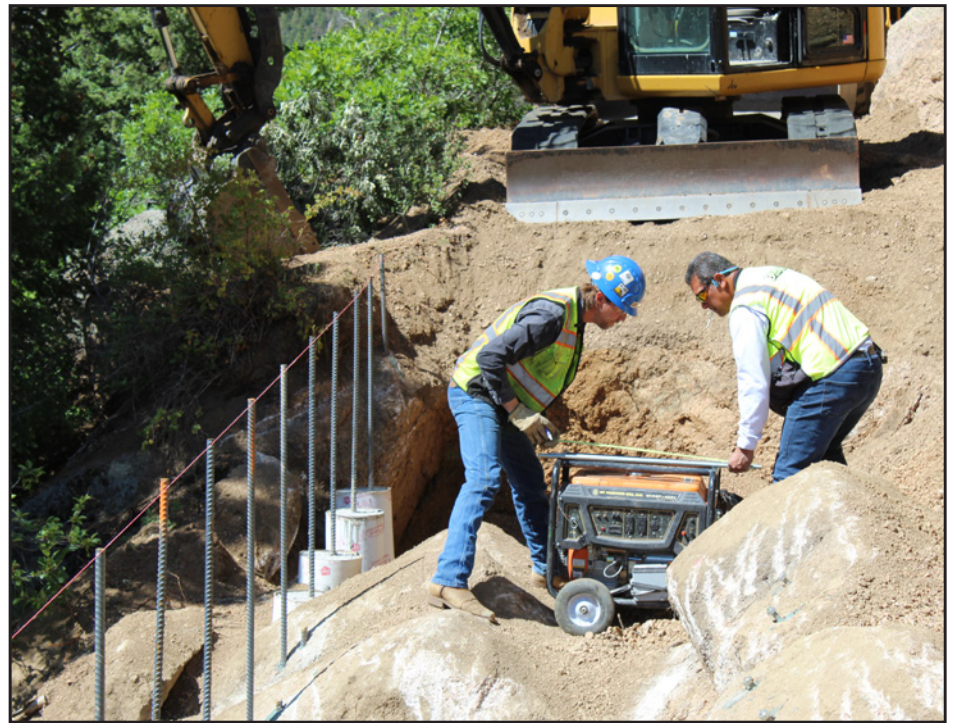
Above: Workers repair a retaining wall along the Reservoir Access Road. Photo by Steve Pate.
