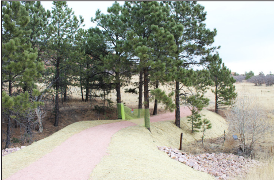
Above: The Santa Fe Open Space (SFOS) is making great progress and is still scheduled to open before the end of the year. Ross Williams, El Paso County community services department park planner, reports that the trail system fencing, and interpretive display are done, and trail and entrance signs are being worked on. Photo by Steve Pate
