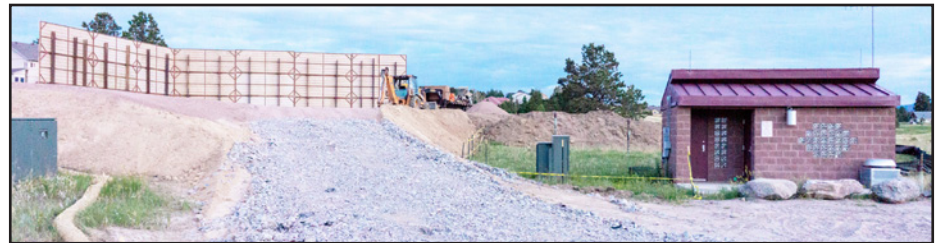
Above: The Woodmoor Water and Sanitation District (WWSD) has installed a sound wall on three sides of the drilling site for Well 22 just south of County Line Road and east of I-25. The new well is just east of a lift station owned by the district. Photo by Jackie Burhans.
