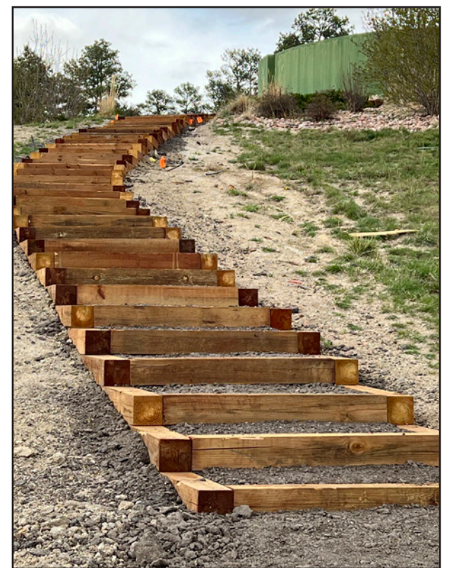
Above: Thirty-nine steps were installed on the St. Lawrence Trail, allowing easy navigation on a steep portion of the district's trail system. The Triview Metropolitan District landscaping crews installed the stairs and plan to overseed the trail area with native grass and replant with trees to further eliminate erosion. The trail connects between St. Lawrence and Penn Central Way and was the access road to B-plant before the development of Promontory Pointe. Photo by Natalie Barszcz.
