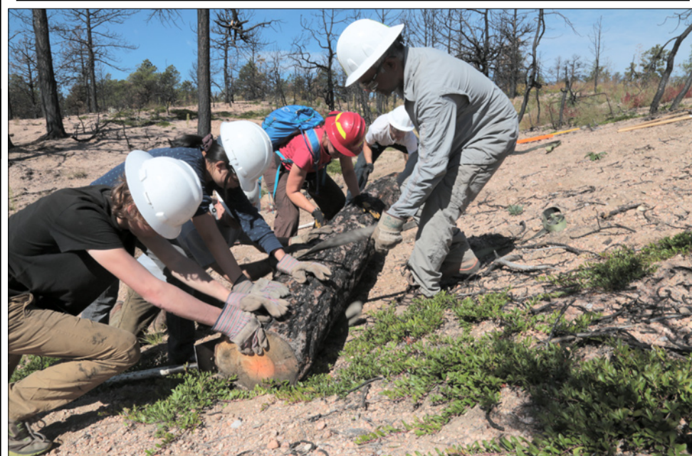
Above: The 2013 Black Forest Fire reduced the ground's ability to absorb rainwater and runoff, presenting the need for anti-erosion practices. On Sept. 13 and 14, volunteers guided by the Rocky Mountain Field Institute used pickaxes, sledgehammers, and saws to install log erosion barriers (LEBs) in Black Forest Regional Park. LEBs allow rainwater to run downhill in wide sheets instead of channeling into deep rills that erode sediment and wash it downstream, clogging drainage ditches and washing out roads. Volunteers also planted grass seed to promote slope stabilization. See www.rmfi.org for more information. See also www.blackforesttogether.org to volunteer to help Black Forest landowners with continuing cleanup work on their properties after the fire. Photo by George Lee. See additional photos on page 23.
